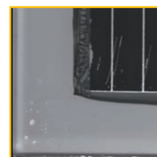
Bubbles in Butyl Sealing
